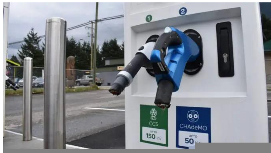
Electric vehicle charging station with severed cables.
